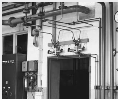
Monitoring for grease and oil ingress in two separate condensate return lines
